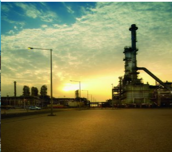
Sasol Qatar 35,000 BPD Gas to Liquids (GTL)
